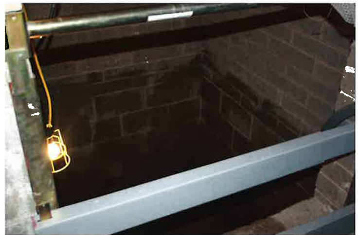
Elevator pit flooded by ground water seepage
