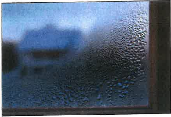
Condensation on the inside of a window-pane.
