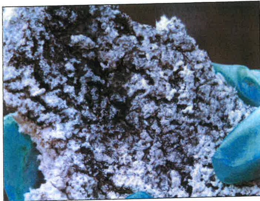
Mold growing on a piece of ceiling tile.
