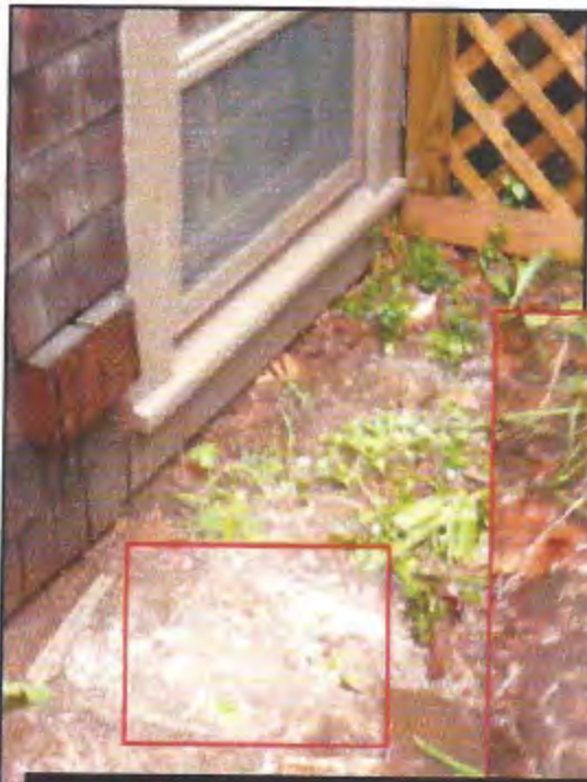
FLOODING BY THE FOUNDATION CAN OVERFLOW INTO THE BASEMENT OVER THE FOUNDATION WALL.
