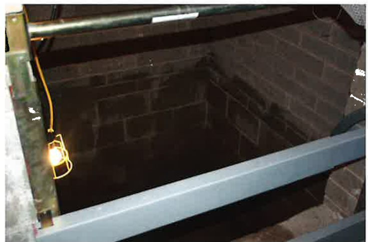
Elevator pit flooded by ground water seepage
