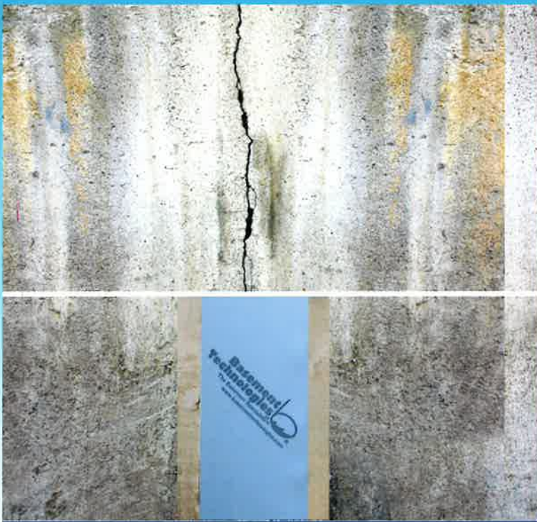
Poured foundation warranted wall seepage solution.
