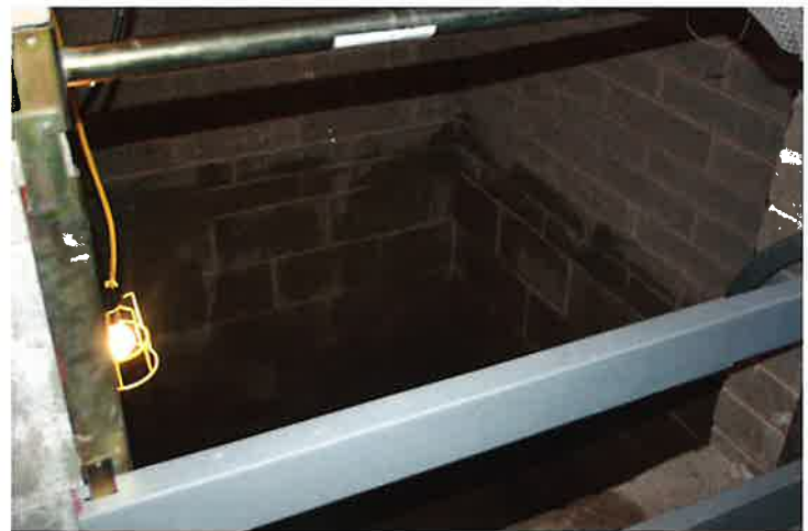
Elevator pit flooded by ground water seepage
