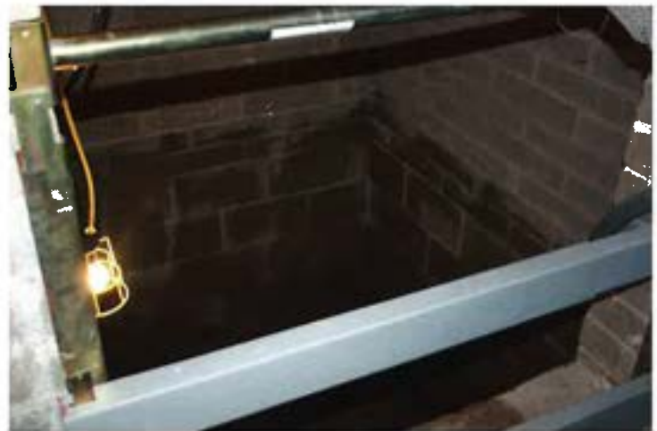
Elevator pit flooded by ground water seepage
